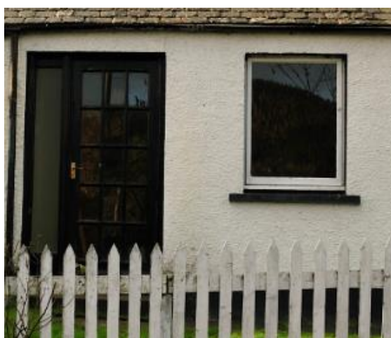
Fig. 68 Inappropriate replacement door and window
