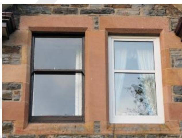
Fig. 69 Inappropriate replacement windows
