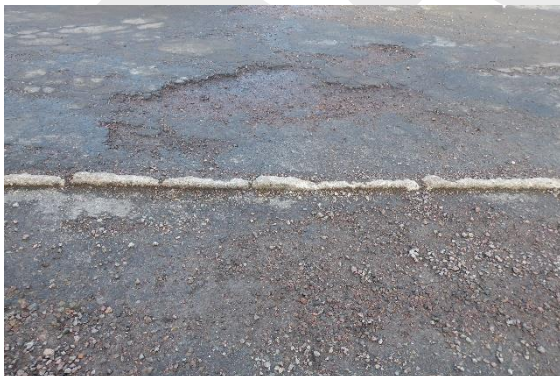
Damaged footpath and car park finishes in need of repair / replacement in Burnfield Avenue.
