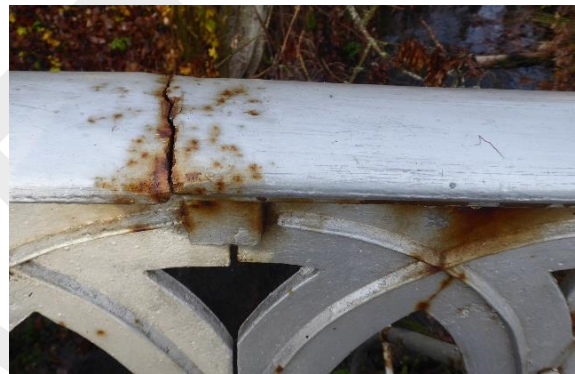
Iron railings on Kyntra Bridge, and the adjacent ornate drinking fountain are in need of minor maintenance.
