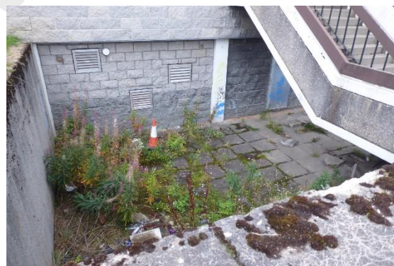
Telecoms building's external light wells and boundary walls in poor condition.
