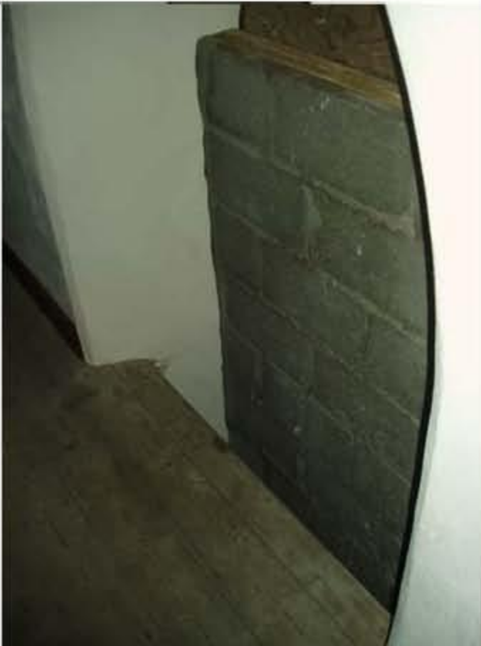
13 - gap between upper balcony wooden floor and window
