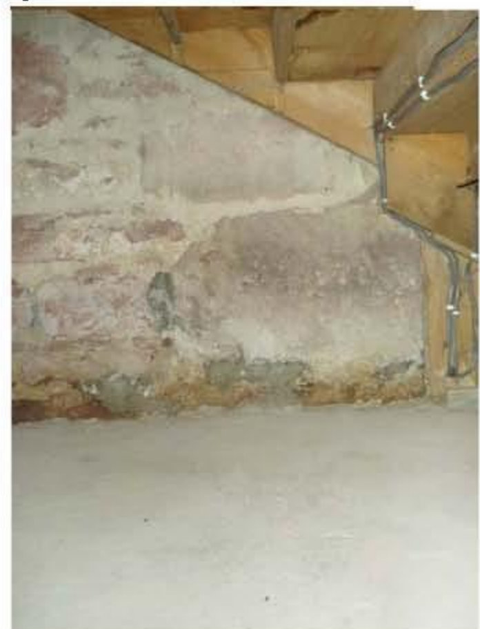
16 - stone work and cement floor under stairs in base of NW tower
