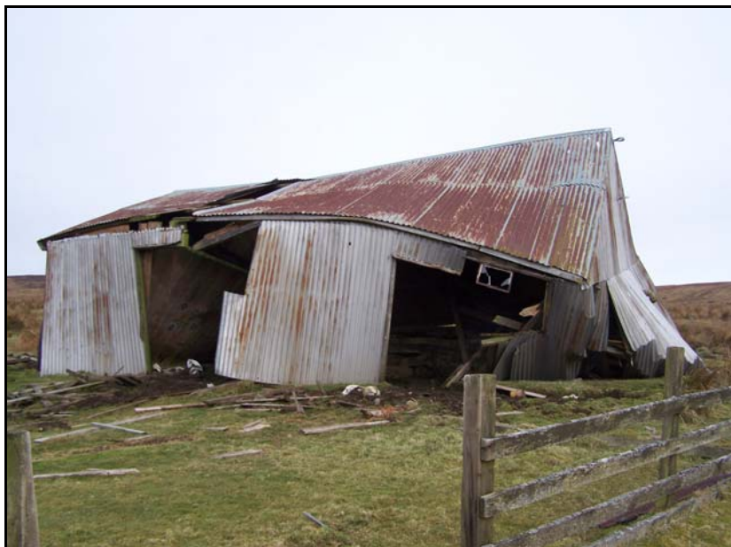
Plate 1: Feature 1 – Collapsed sheep shearing shelter (from S).
