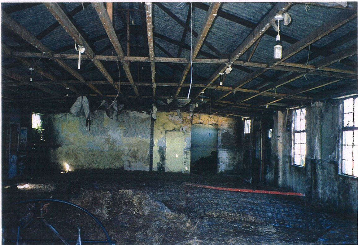
Photograph No. 36C Looking NW at interior of S end of Building C.3
