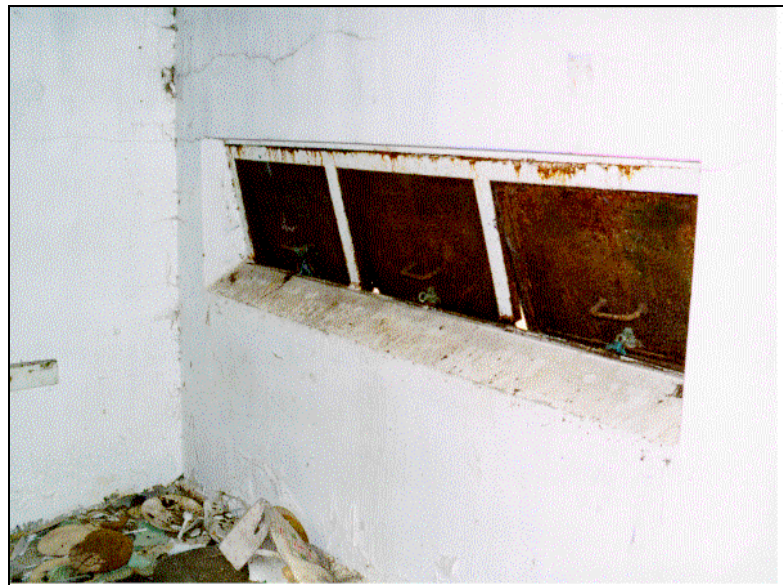
Photograph W17: Interior view of chutes in decontamination centre
