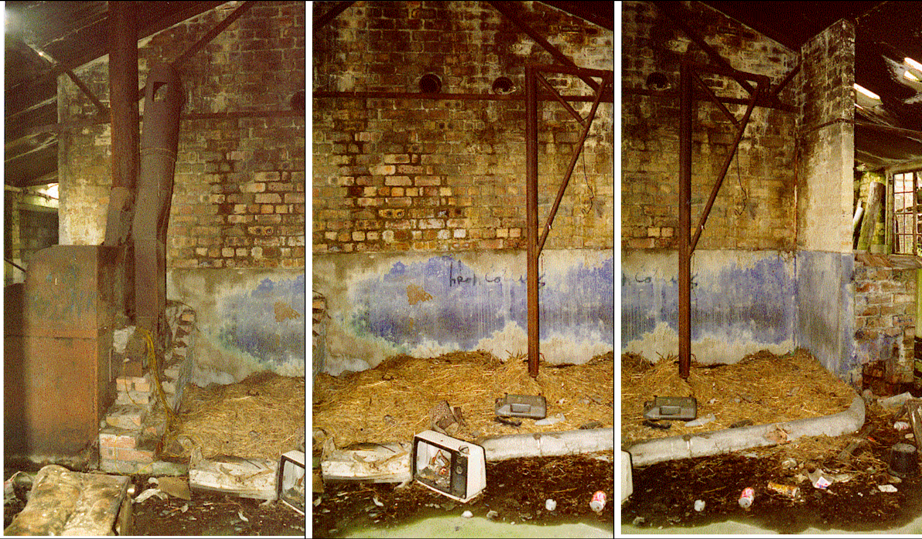
Panorma W53/W54/W55: internal view of hospital block FEARN AIRFIELD – PHOTOGRAPHIC SURVEY AREA H
