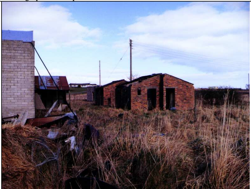
Photograph A11: Ablutions blocks adjacent to torpedo shed FEARN AIRFIELD – PHOTOGRAPHIC SURVEY AREA A/G
