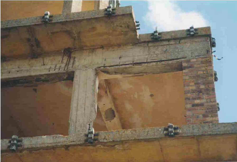
Photo 3 Control Tower concrete deterioration of 2 nd floor structure viewed from the south
