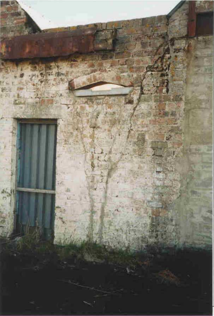
Photo 7 Torpedo sheds Cracked brickwork on west gable wall at junction with nissen nuts
