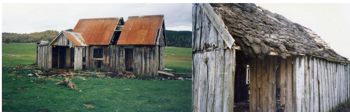
Sleeper House, 1995, and 1997, roof blown off and turves exposed.
