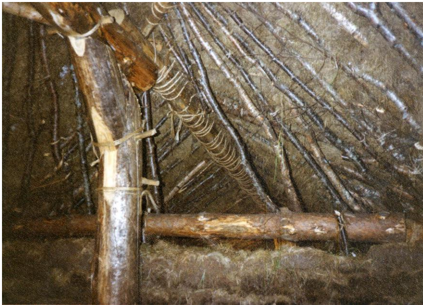
Roof detail showing a jointed cruck, roof spars and purlins with turf divots on top. Highland Folk Park 1999
