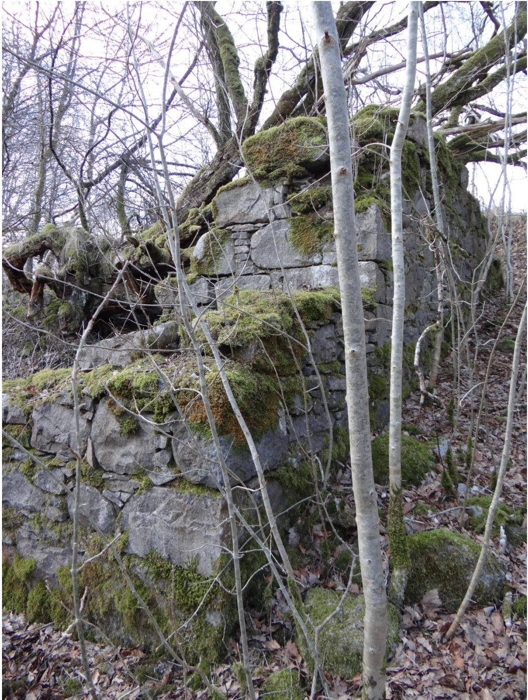
10 - South eastern corner of the eastern section, view from the south east
