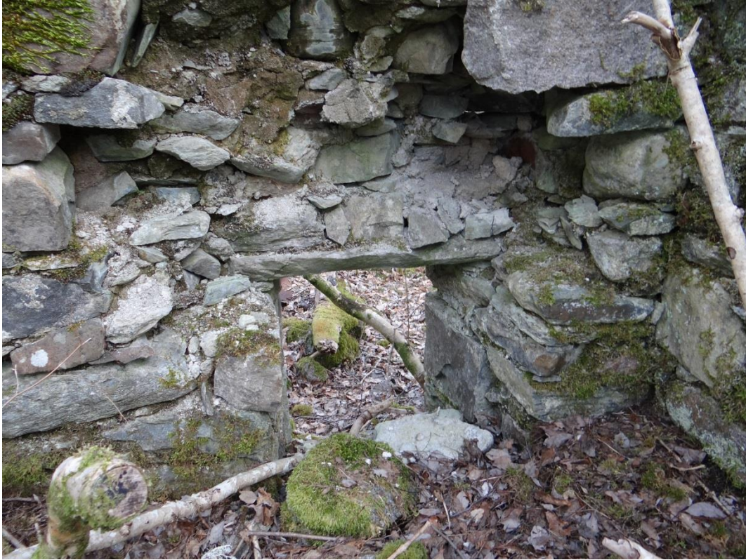
22 - Close up of the window in the eastern wall, view from the interior, facing east
