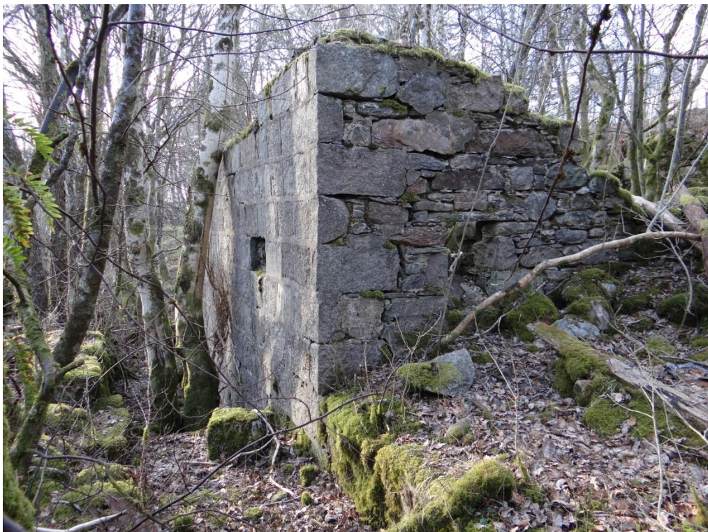
12 - The main wall and channel of the water wheel, viewed from the east
