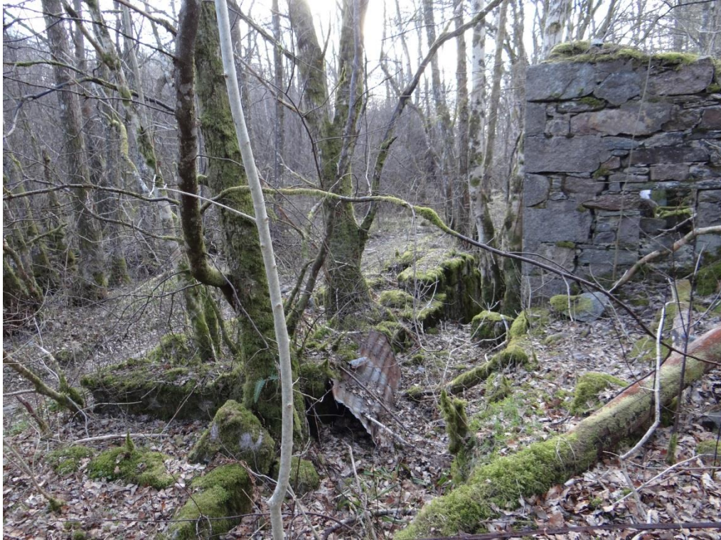
11 - The channel running towards the main southern wall, view from the east, facing west
