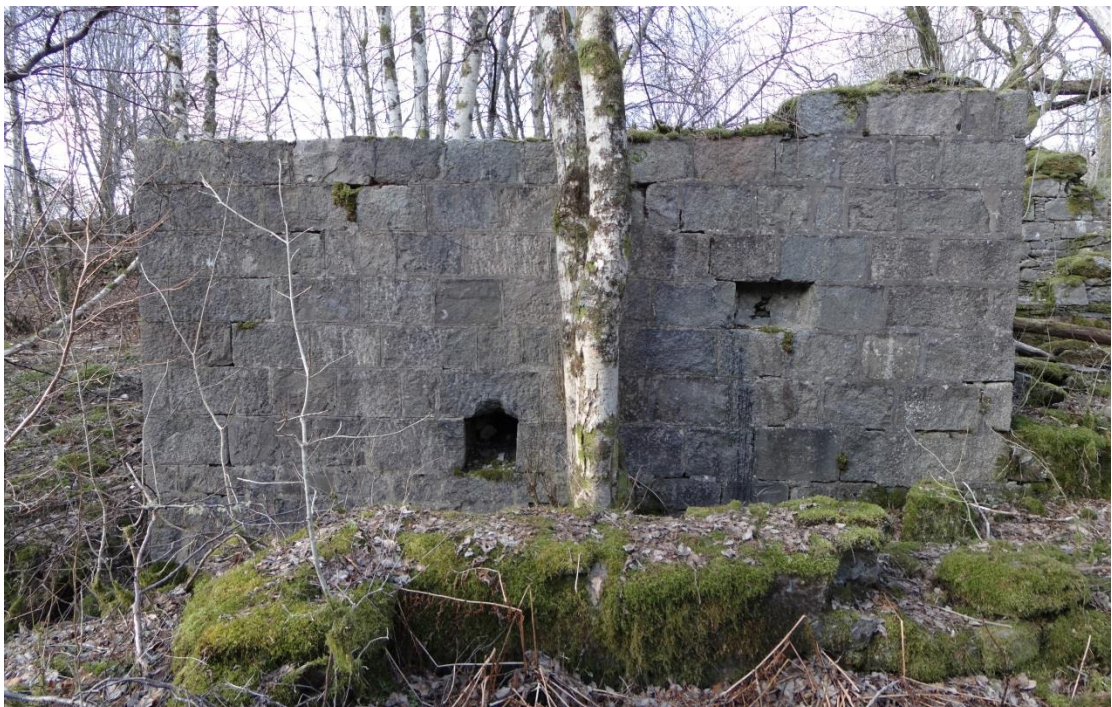
28 - View of the exterior, main, southern wall where the water wheel would have been located, facing north
