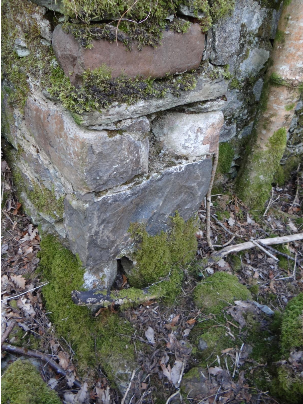
15 - Detail of the northern side of the most northerly gap in the western wall, view from the south west facing north east
