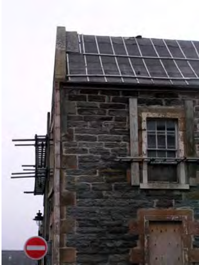
Bulging masonry at the southeast corner
