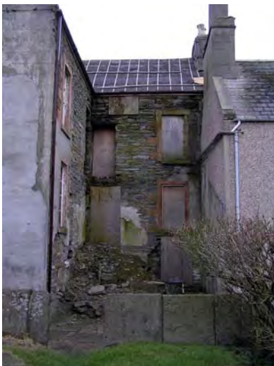
The re-entrant to the rear of the property following the demolition of the stair tower
