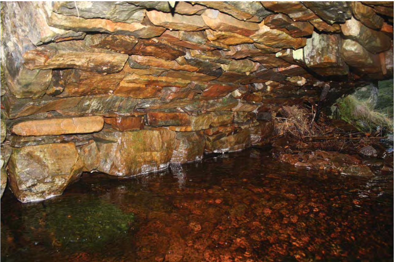
Plate 4: Bridge 007, general view of the underside of the bridge to the north side, from the north-west
