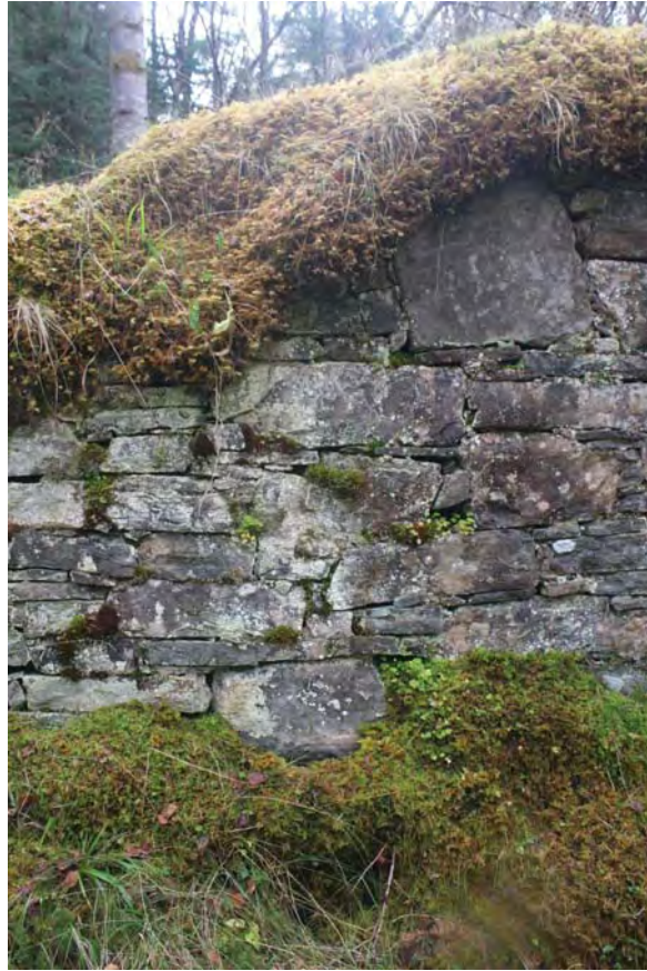
Plate 31: Bridge 009, detail of the north side showing the missing pinnings and heavy moss and lichen growth to the abutment wall on the east side
