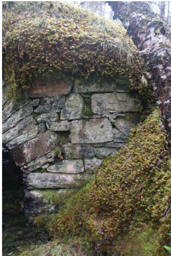
Plate 30: Bridge 009, detail of the north side showing the missing pinnings and failed pointing to the abutment wall on the west side
