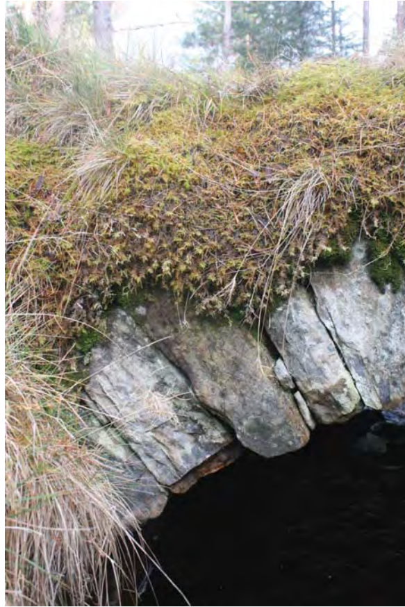
Plate 19: Bridge 007, detail of south side showing the slipped voussoirs and loose pinnings on the west side
