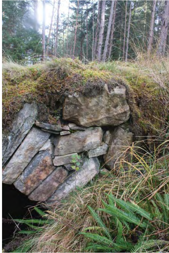
Plate 21: Bridge 007, detail of the south side showing the displaced spandrel stones and loose pinnings on the east side
