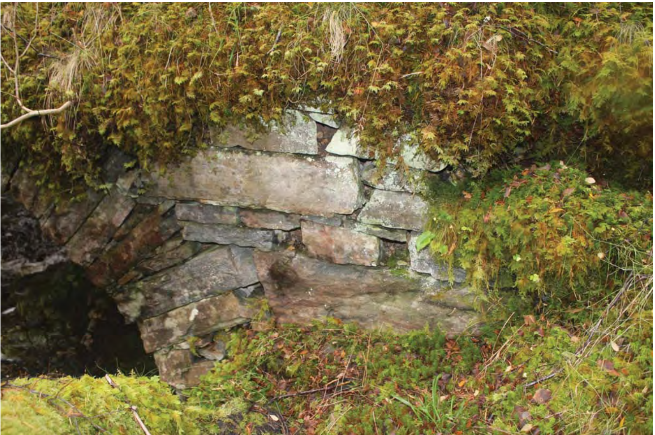
Plate 28: Bridge 009, detail of the south side showing the deep cavities and missing pinning on the abutment wall on the east side
