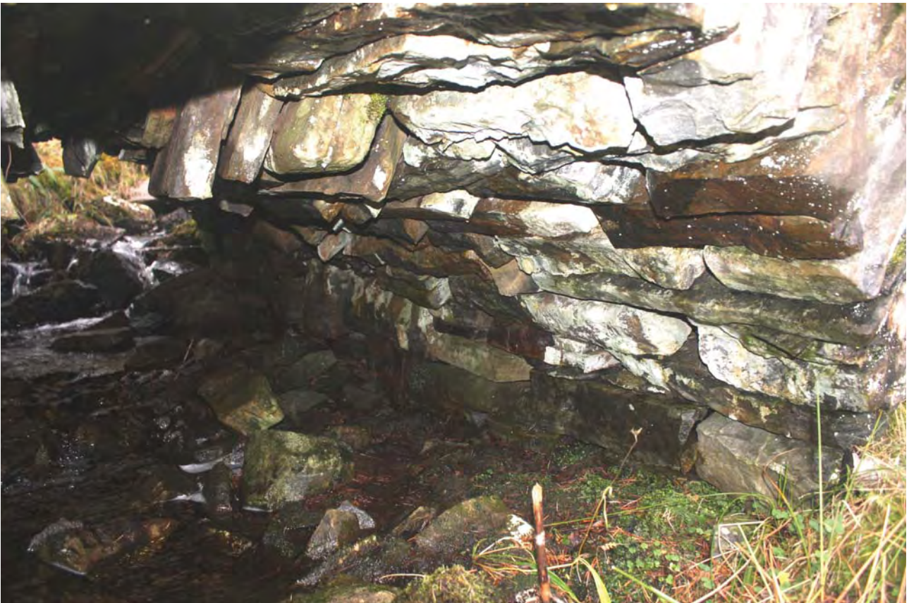
Plate 8: Bridge 008, general view of the underside of the bridge on the west side from the north-east
