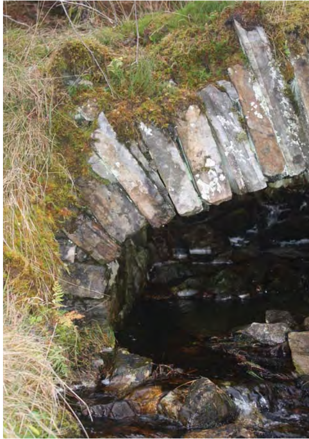
Plate 25: Bridge 008, detail of the north side showing the slipped voussoir stones to the east side
