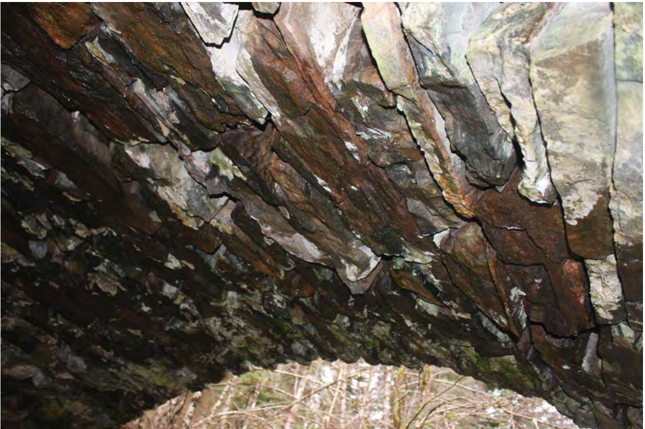
Plate 14: Bridge 009, general view of the underside of the bridge form the north
