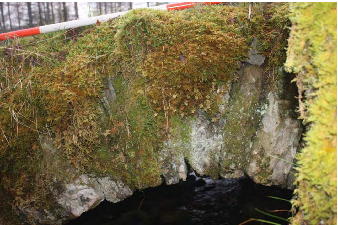
Plate 24: Bridge 008, detail of south side showing voussoir stones on the west side
