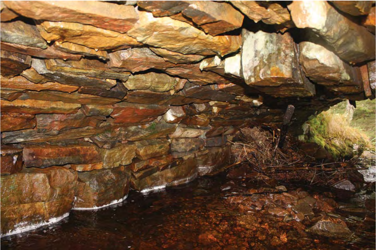
Plate 23: Bridge 007, detail of the underside of the bridge showing the partially blocked water course and slipped arch barrel voussoirs to the underside of the arch
