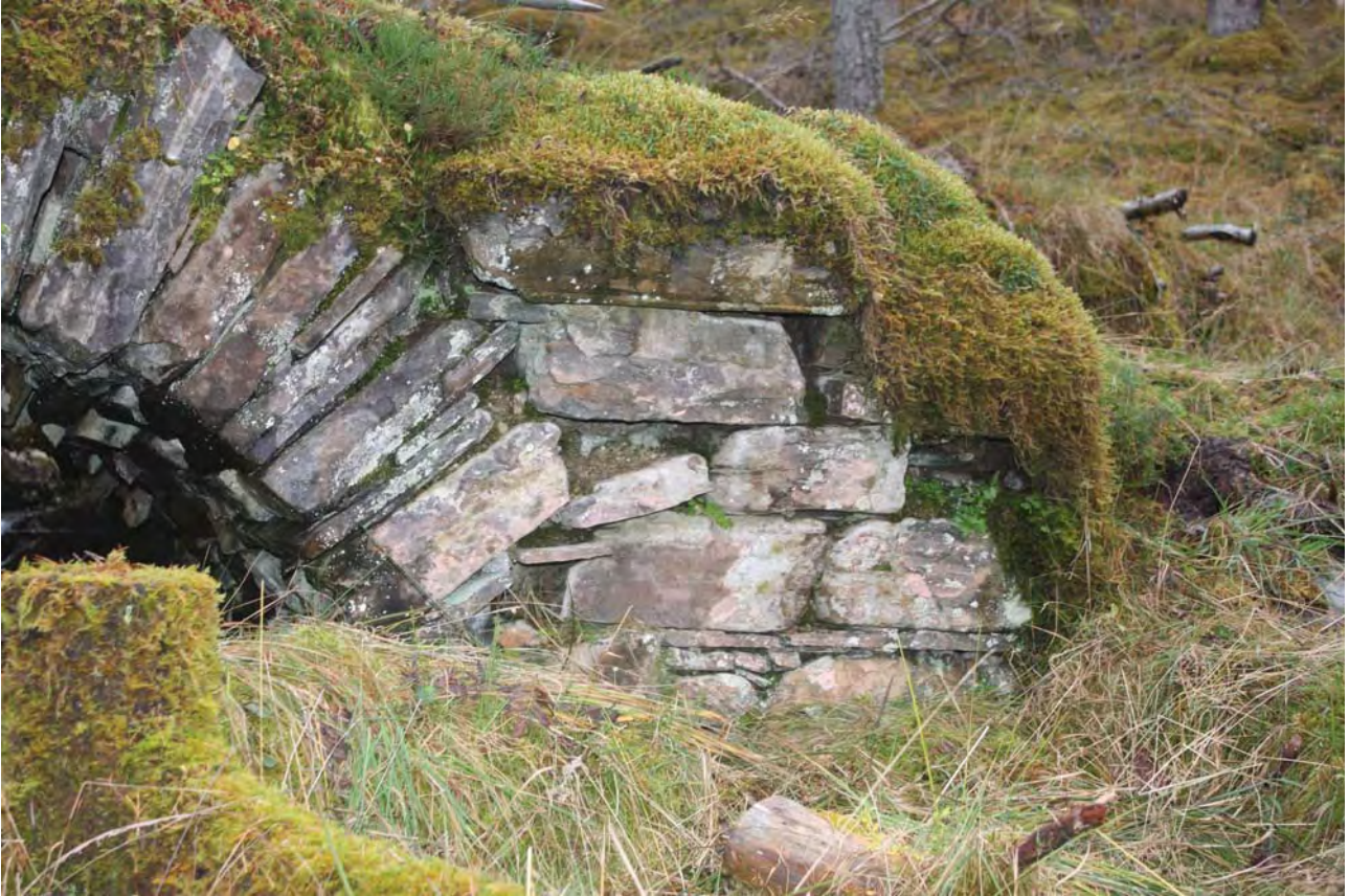
Plate 27: Bridge 008, detail of the north side showing the displaced and loose spandrel stones to the western abutment wall
