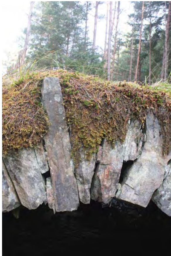
Plate 20: Bridge 007, detail of the south side showing the slipped voussoirs and badly slipped voussoir at the head of the arch
