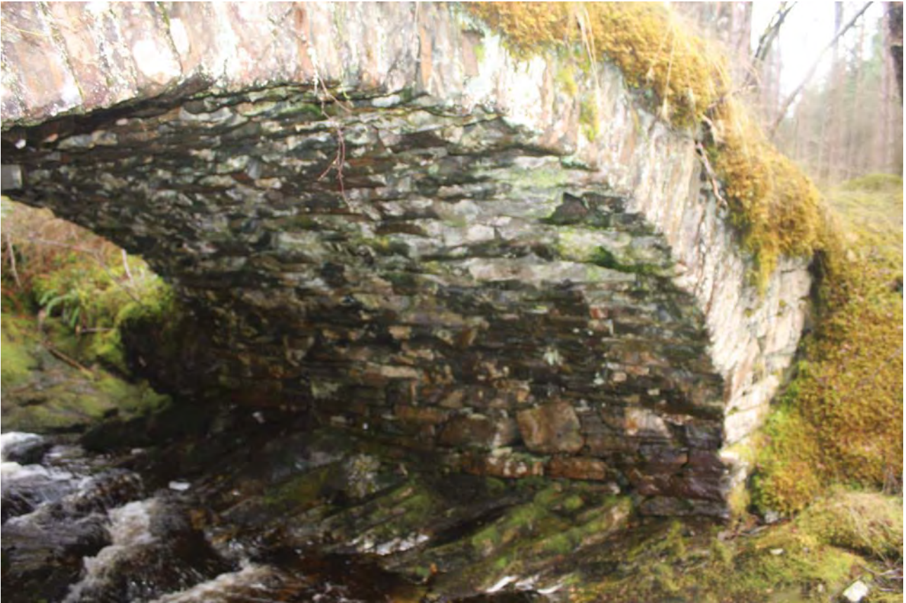
Plate 13: Bridge 009, general view of the underside of the bridge on the east side from the north-east
