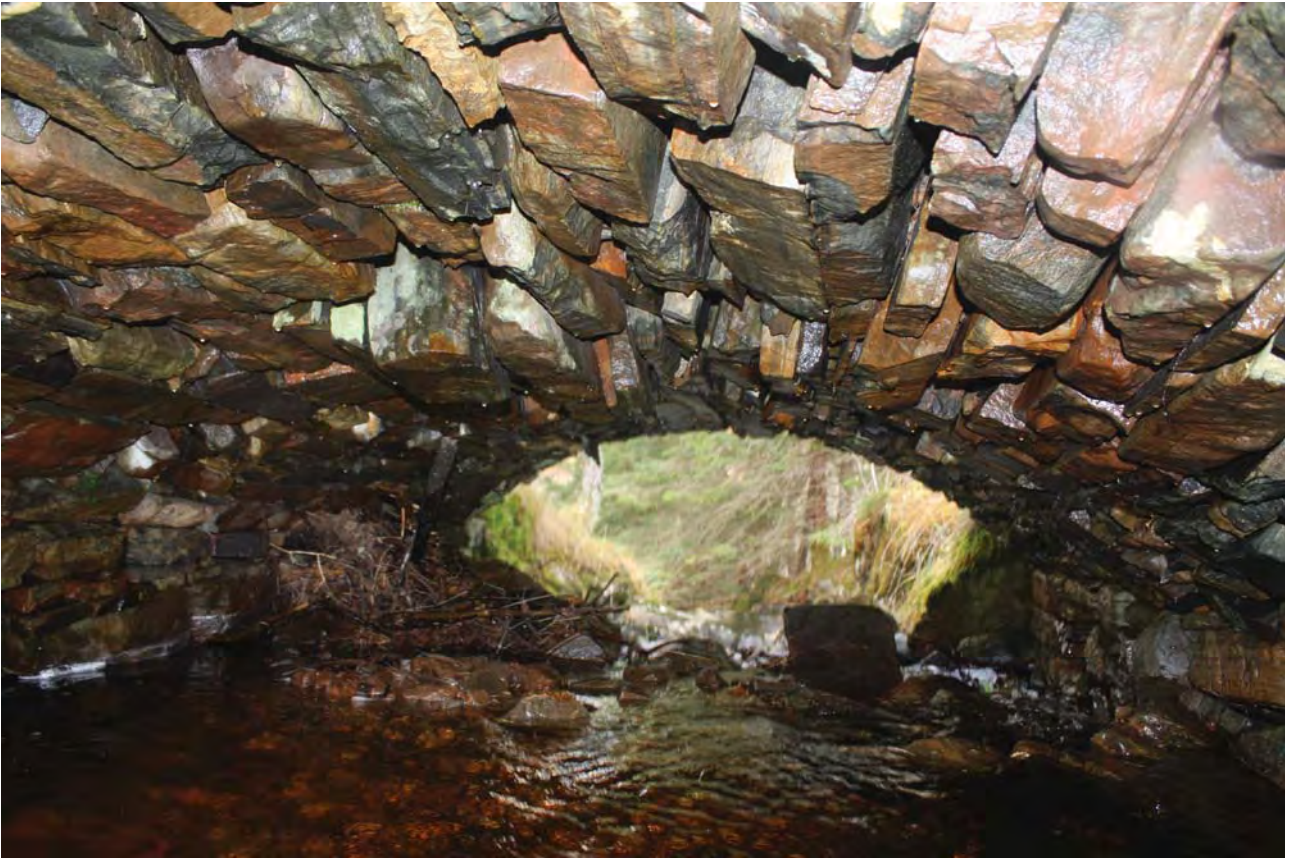
Plate 5: Bridge 007, general view of the underside of the bridge, from the north
