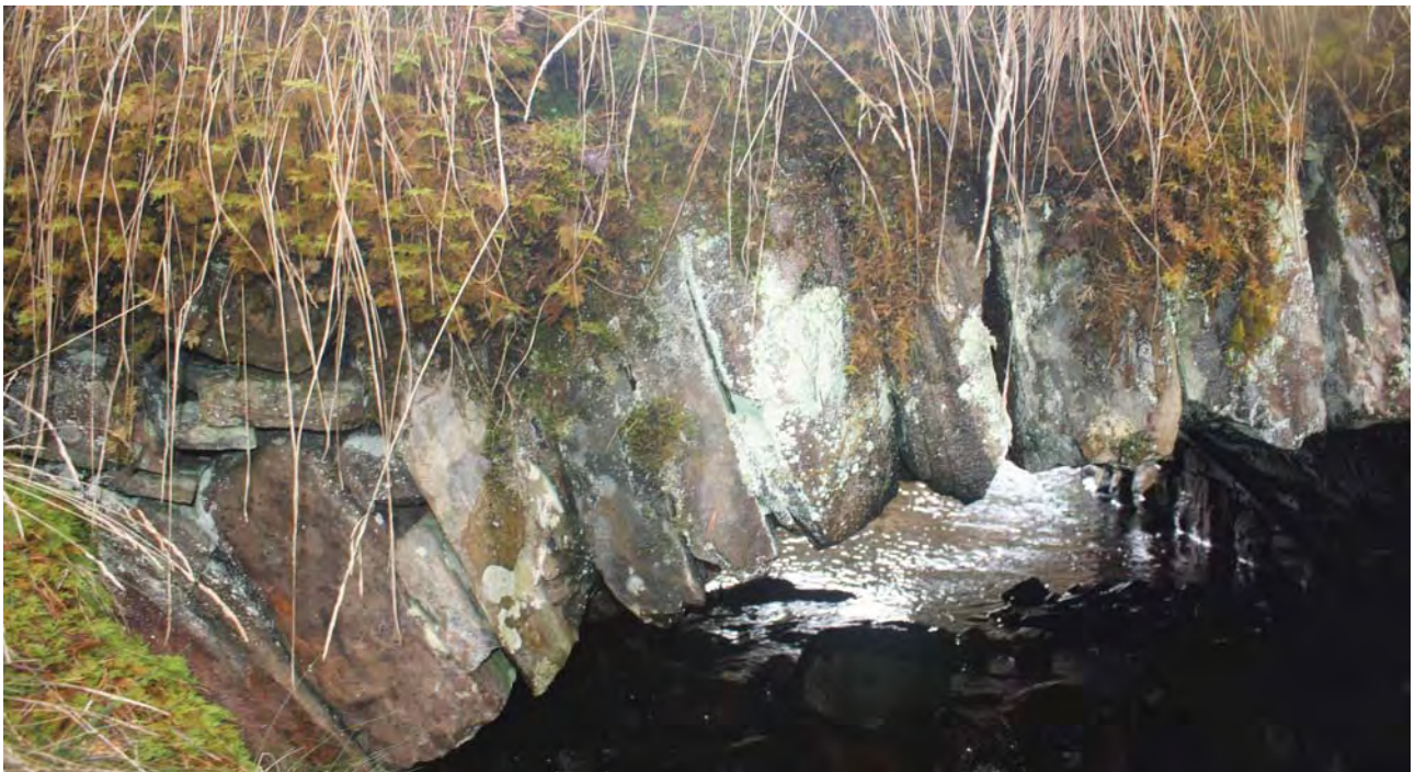
Plate 22: Bridge 007, detail of the north side showing the slipped voussoirs
