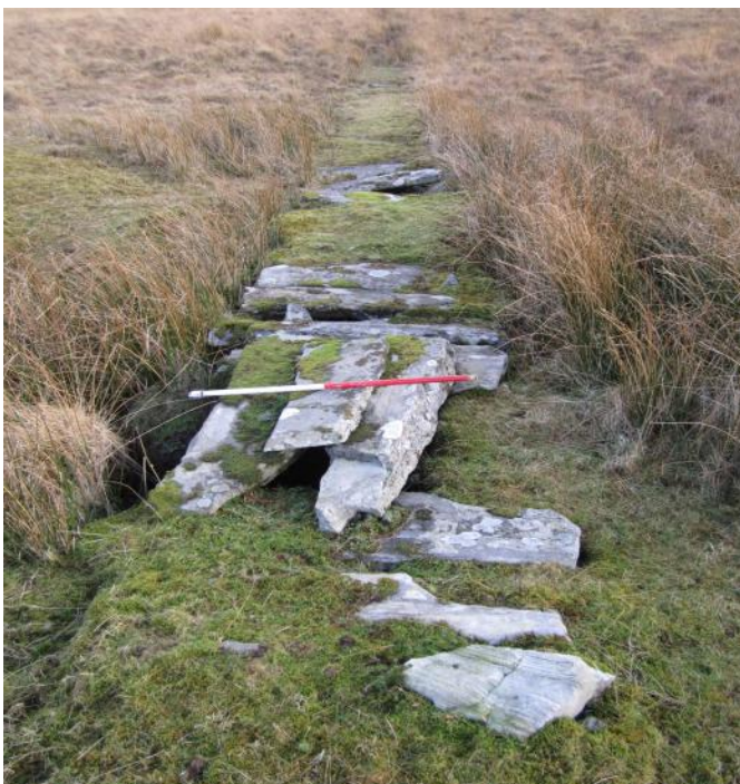
Wp 24 Exposed stone slabs over field drain NM 63268 85331
