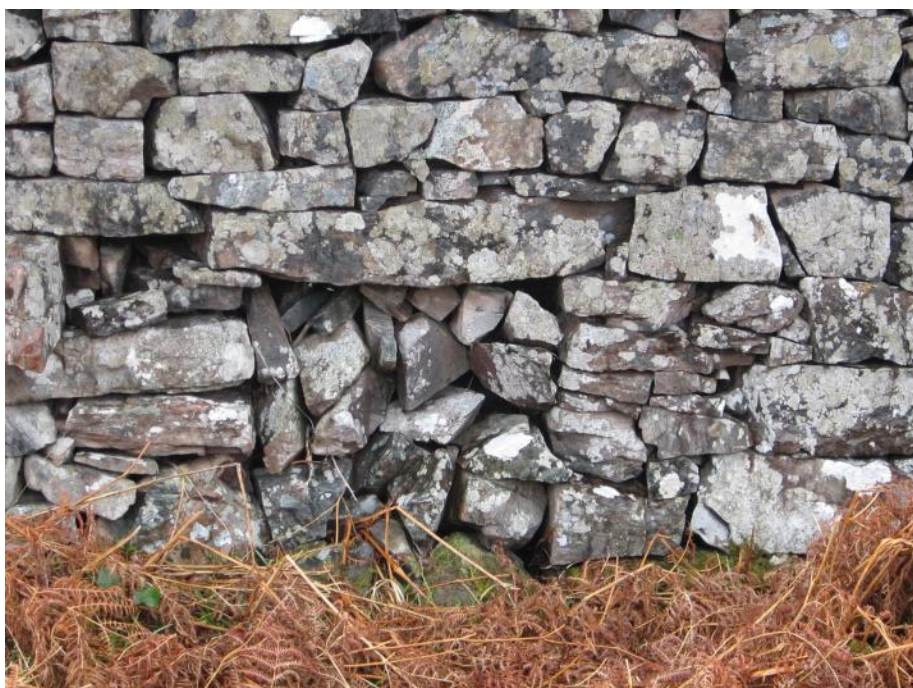
Wp 15 Detail of the Sheep fank showing blocked sheep creep at NM62551 84713
