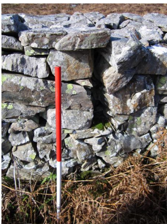
Wp 8 A Ruin c. 7x4 showing close up of cruck slot at NM 82680 83397
