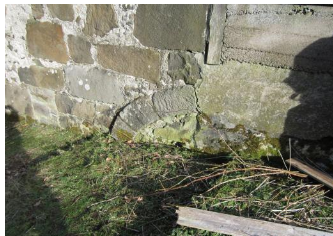
Wp 42 Curved stone work on Mill by covered laid NM 64595 85001
