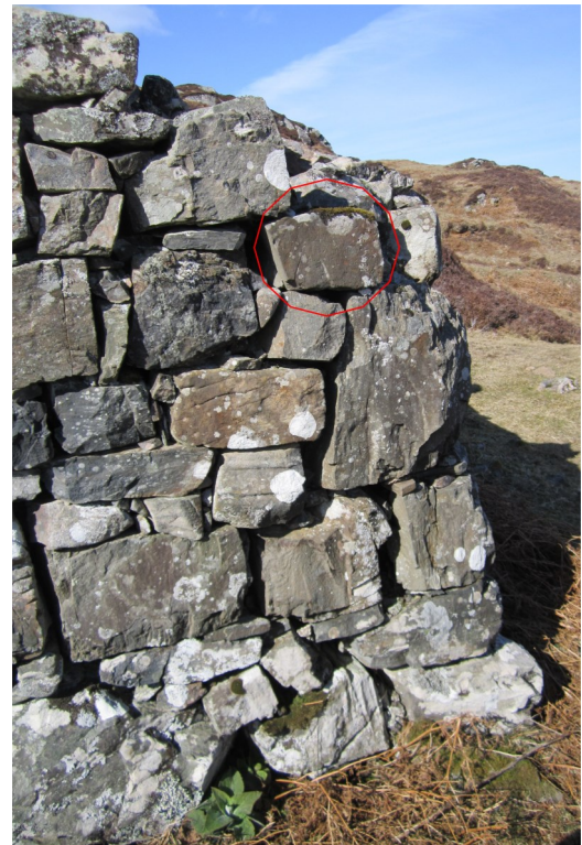
Wp 10 View of NE corner of building showing the position of the incised stone
