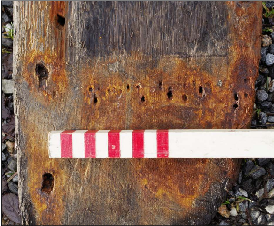
Plate 12: An example of small fastenings visible on the scarph joints (T-16)
