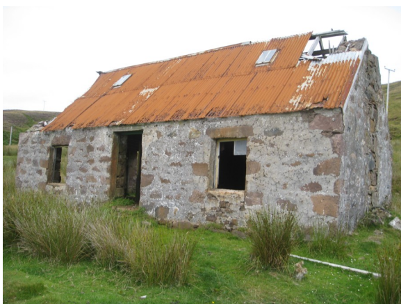
1 NG 74112 87021 63m ruined house
