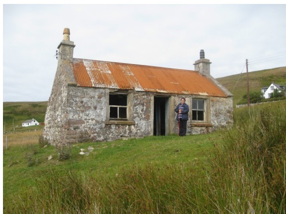
13 NG 74094 86839 53m ruined house
