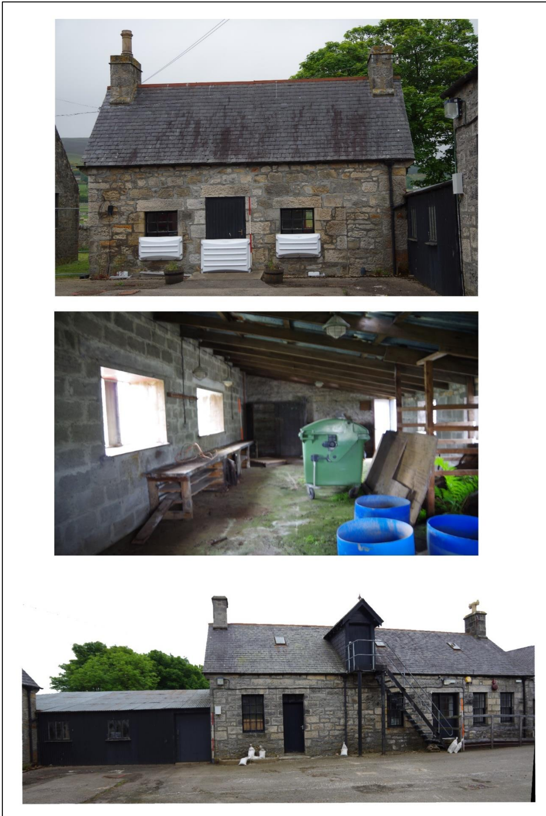
Figure 32 – (from top) SW facing elevation of ANC1, the interior of ANC2 and the west facing frontage of ANC2 and ANC3. Scales 2m
