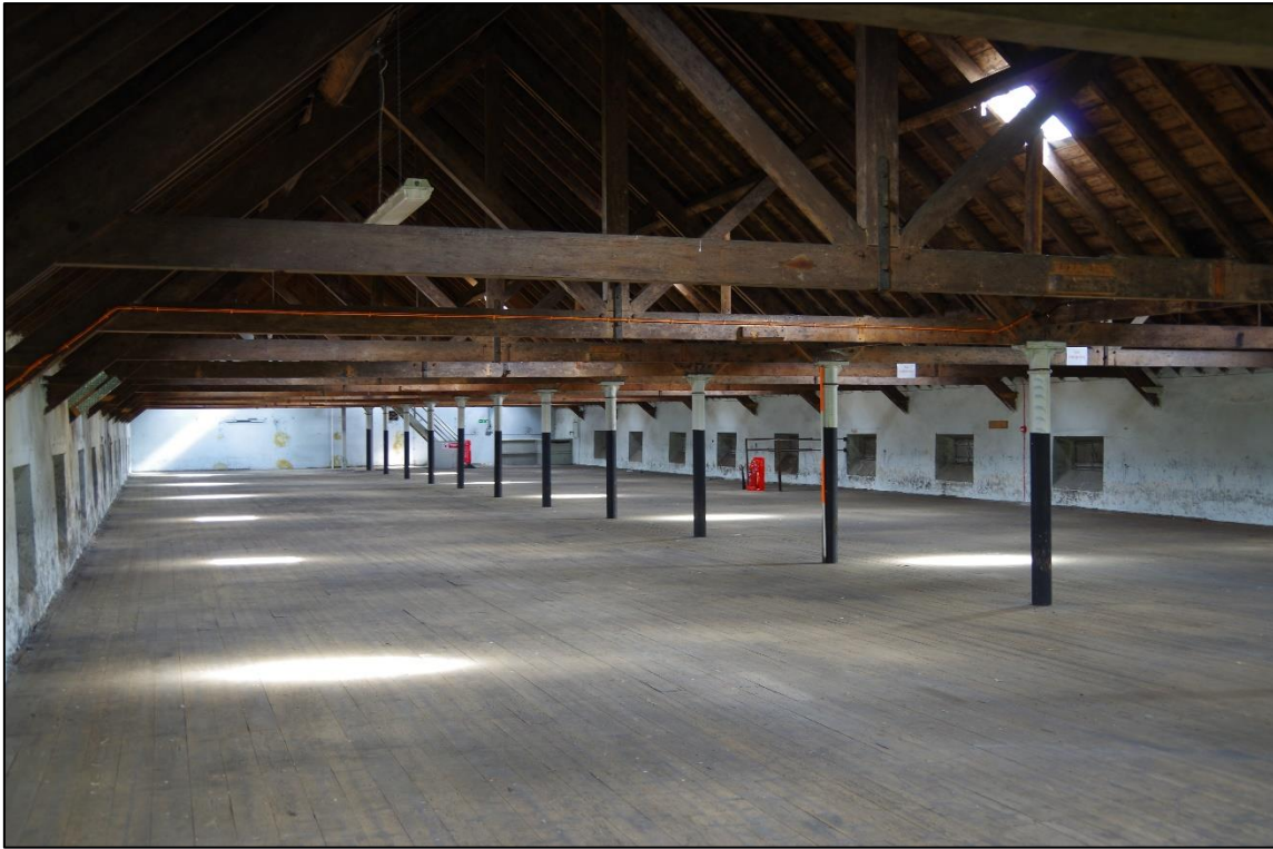
Figure 11 – The interior first floor of the Cooperage building facing NE. Scale 2m
