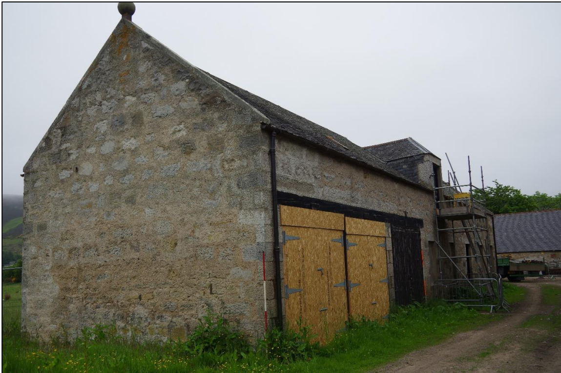
Figure 13 – The south and east facing elevations of the Stable Block. Scale 2m
