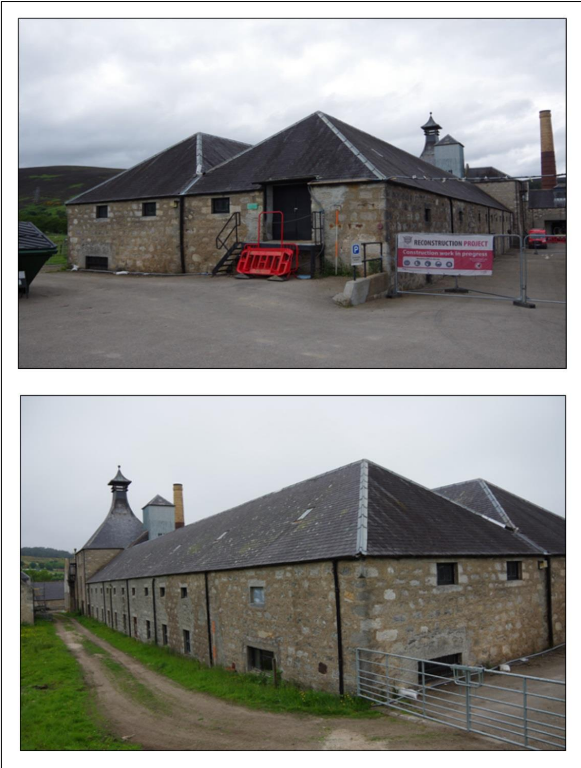
Figure 8 – The south gable end and W facing elevation of the Cooperage building. Facing N and NE. Scales 2m
