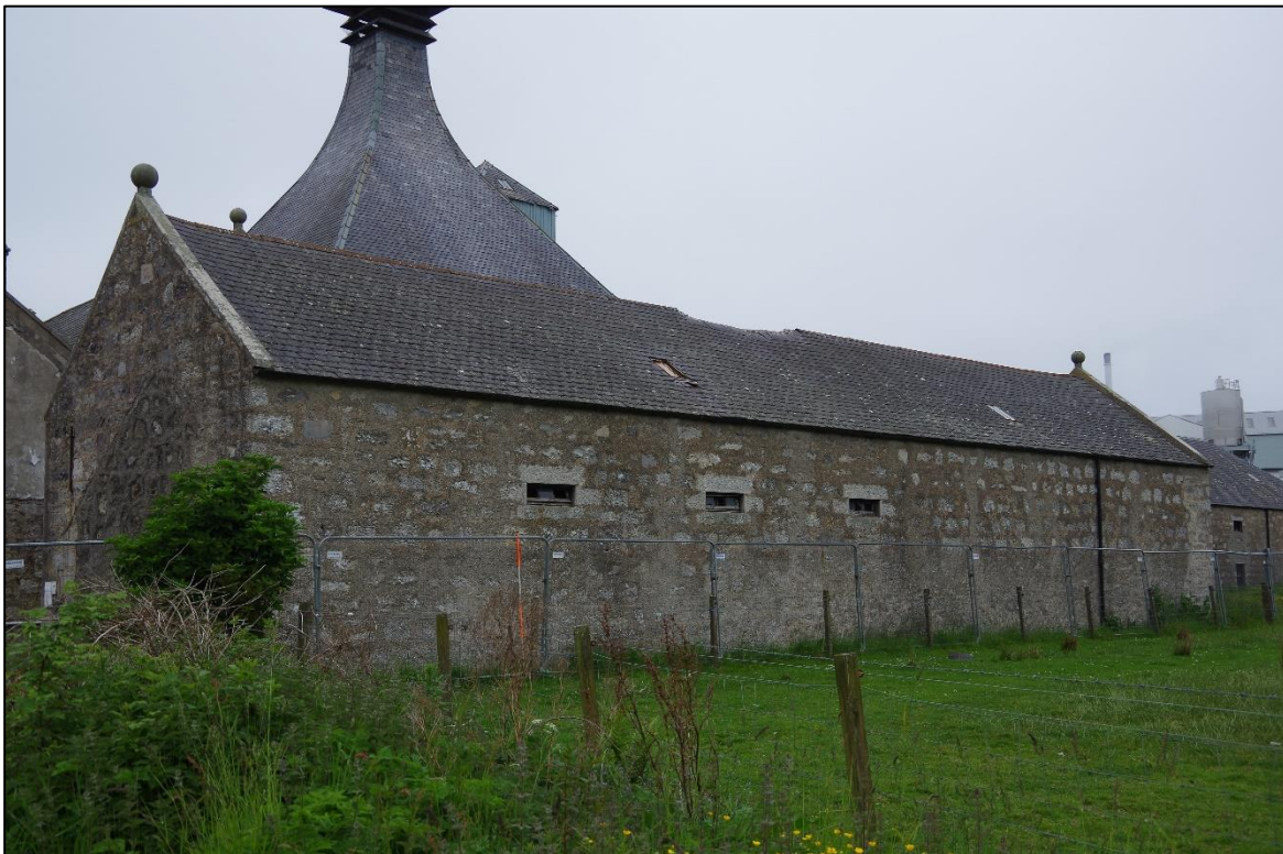
Figure 14 – The west elevation and north facing gable wall of the Stable Block. Facing SE. Scale 2m
