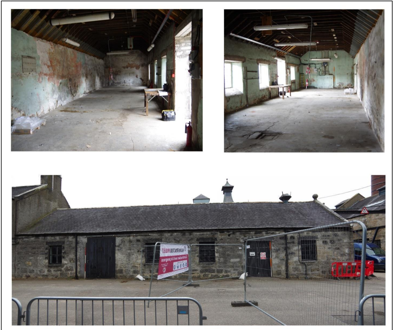
Figure 33 – The E facing frontage and interior of the Stores Building. Scales 2m
