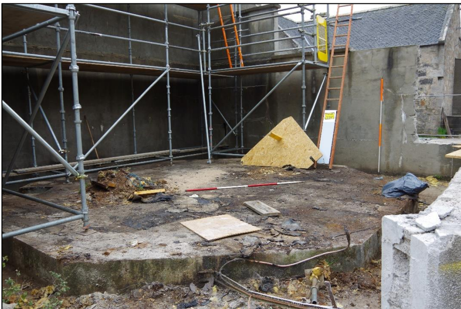
Figure 31 – The foundations of the Oil Bund (recently removed). Facing SE. Scales 2m
