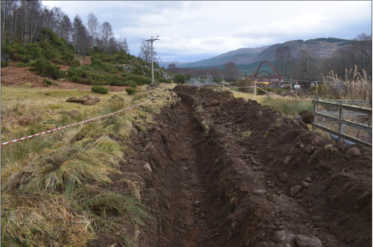
Plate 38: Record image of cable trench from steading at the west end of the site, facing east
