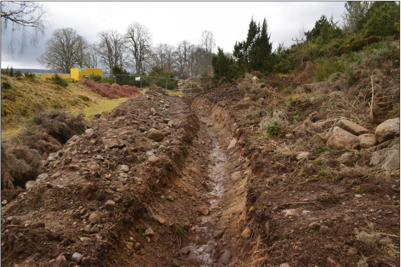
Plate 39: Record image of the east end of the cable trench, facing west
