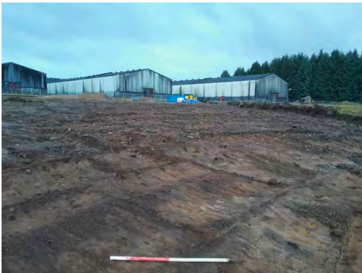
Plate 8: Post excavation of the southeastern corner of the main construction area, showing changing ground levels, facing northwest
