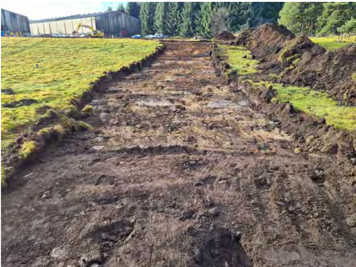
Plate 4: Post excavation of haul road under soil storage bund area, facing west
