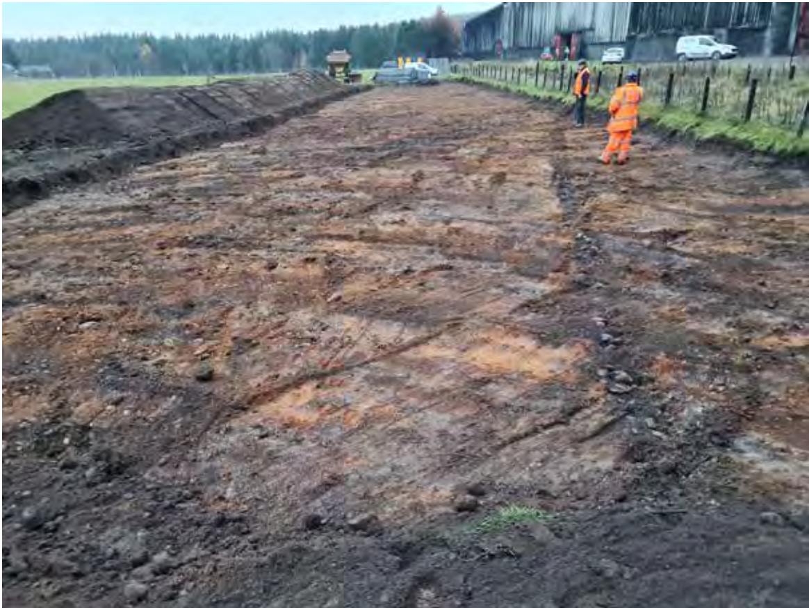
Plate 1: Post excavation of first area in the northwestern edge of the site showing field drains, facing south
