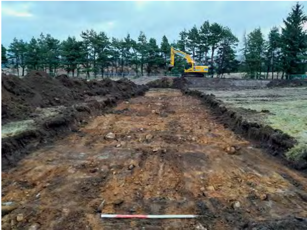
Plate 9: Post excavation of the northern leg of pipe trench route, facing east
