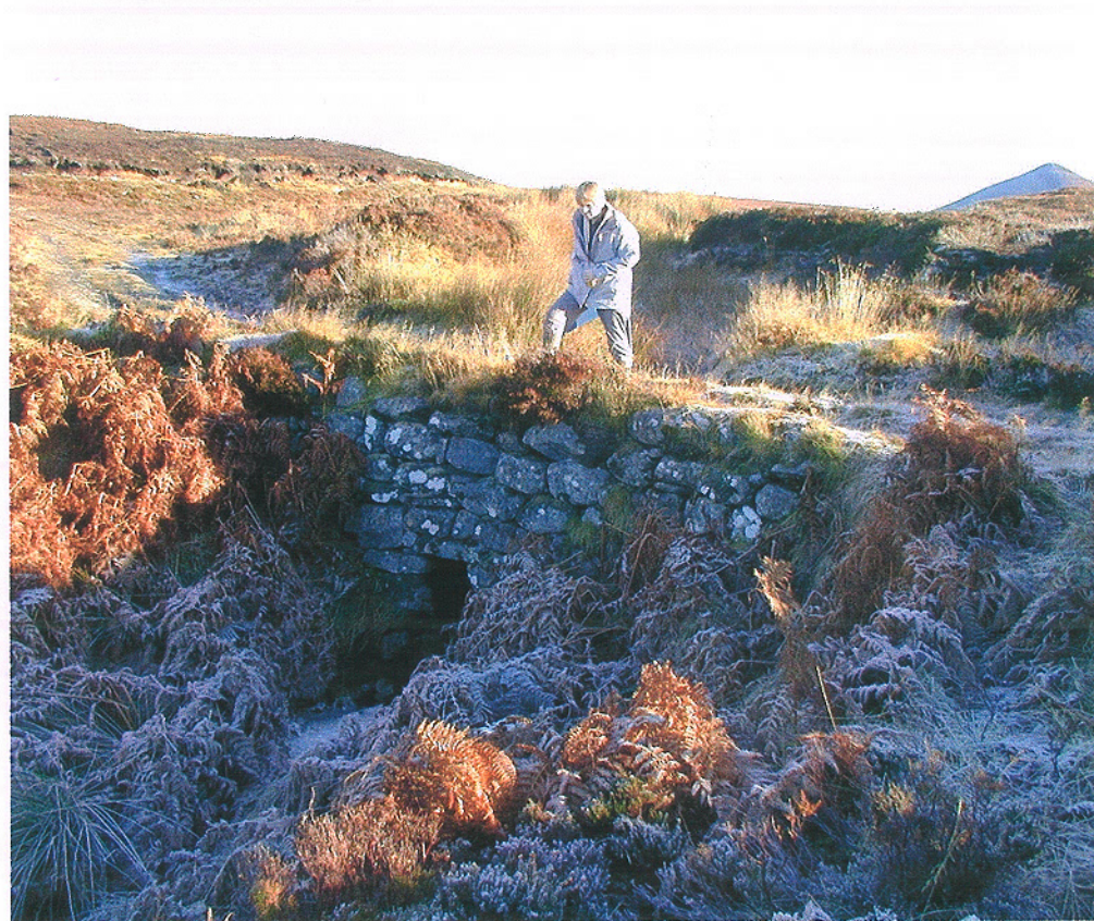
Plate 18. Feature 073. Stone facade to downstream headwall of culvert crossing under the existing access track (Feature 001) on exposed moorland E of Allt a'Mhuilinn. GR 283156 912278
